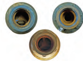
Inlet and outlet of worn pressure regulators.
